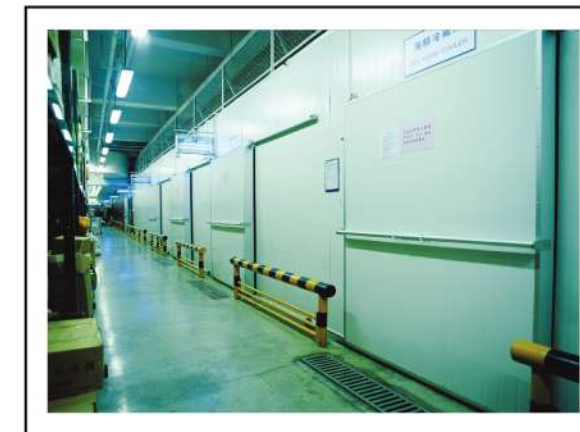
冷藏/冷冻库 Cold Room
