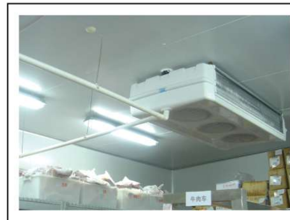
冷库风机 Cold-room Refrigerator
